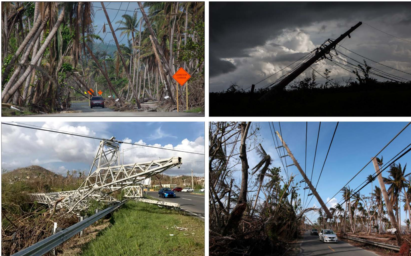
Figure 1. Damaged Power Lines and Electricity Grid Infrastructure in Puerto Rico in November 2017 after Hurricane Maria
