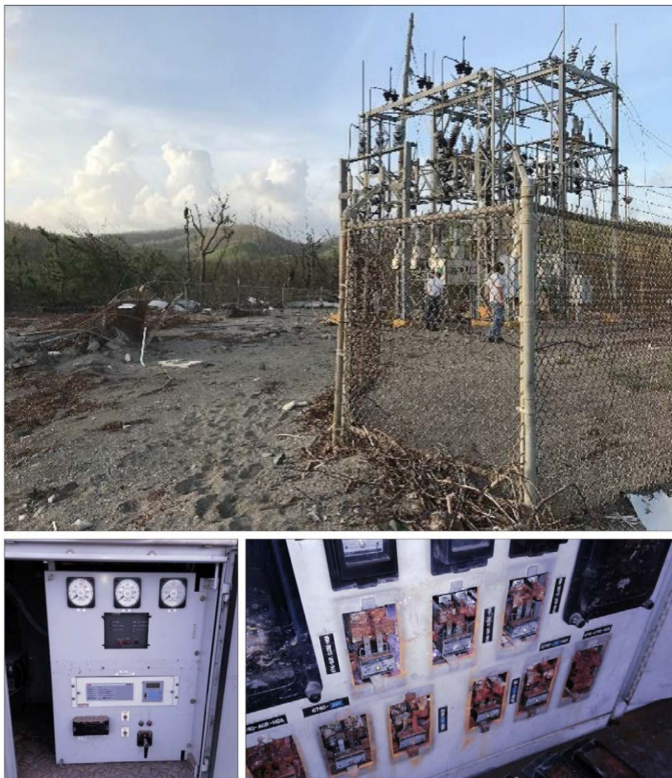
Figure 3: Evidence of Damage and Flooding from Hurricanes Irma and Maria at Critical Substations in Puerto Rico
